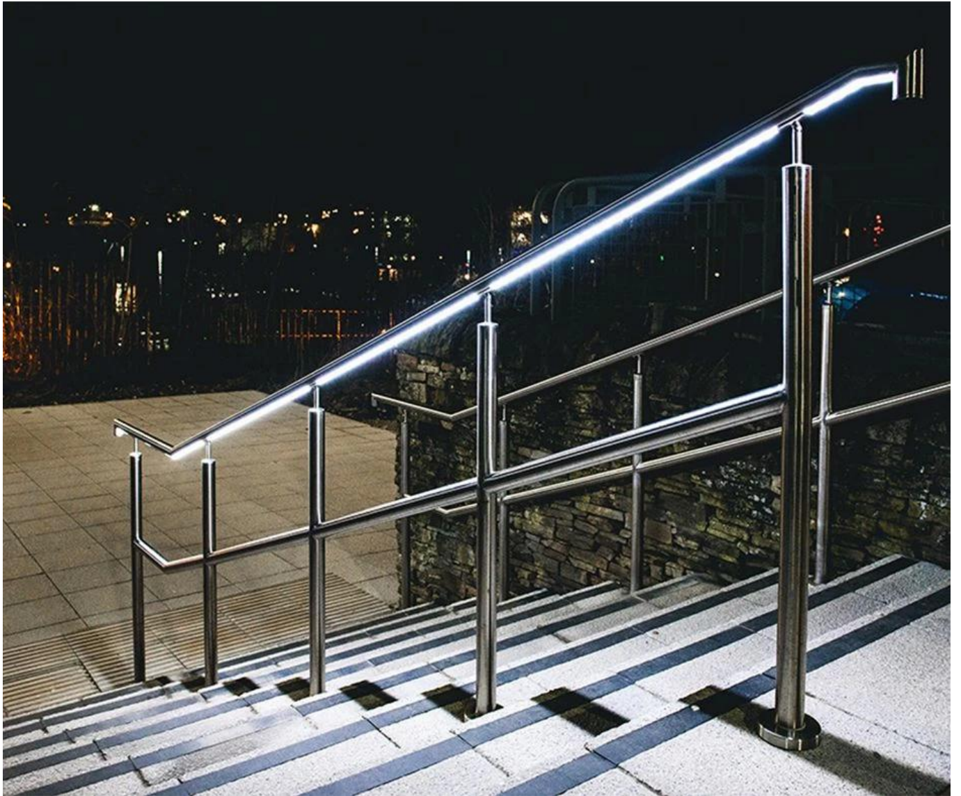
3) Stainless Steel LED Handrails
